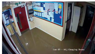
Water in the clubhouse
